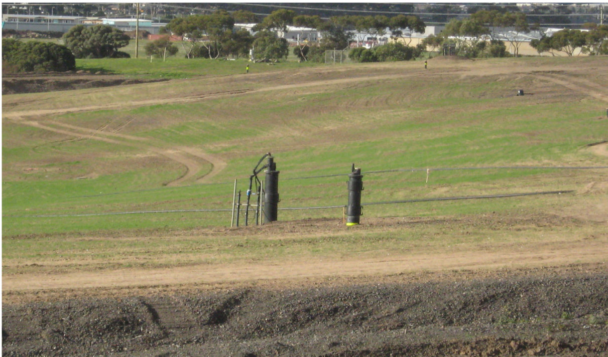
Figure 5: Leachate collection wells on the capped Cell 2A of Stage 2 of the existing landfill
