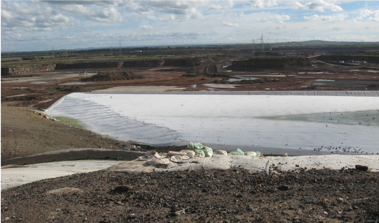
Figure 3: View looking west from Stage 2 (existing landfill), showing the intermediate cover (foreground), the geotextile liner in the base of Cell-2M (in the middle of the photo) and the base of the excavated quarry floor for proposed Cell 3 (top of the photo).
